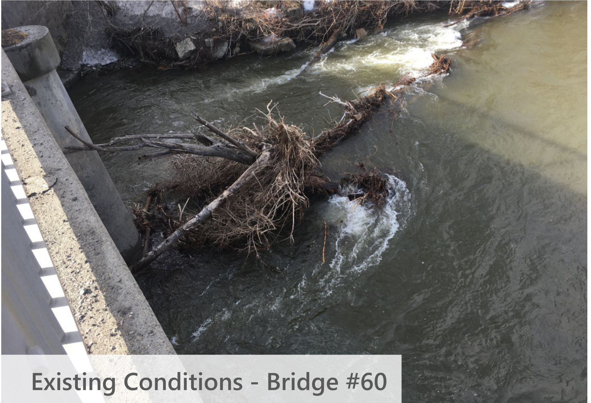
Typical Debris Jams at Pier
